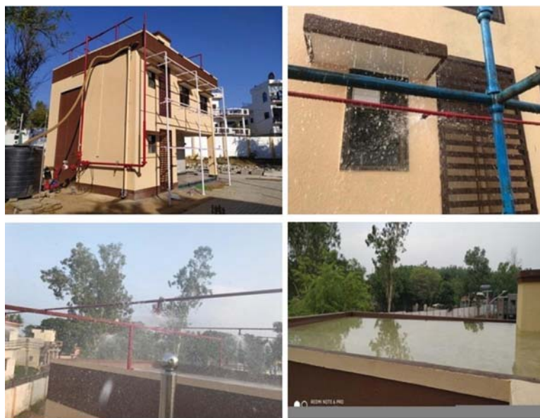
Fig. 2. View of water tightness test setup and actual testing at AAC building.
