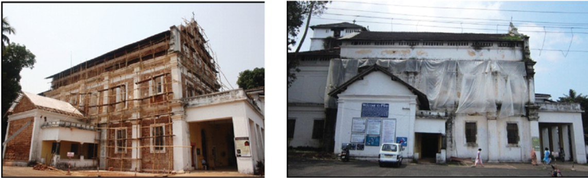
Fig. 1. Nossa Senhora do Pilar church (Goa, India) during and before restoration. Some important architectural details of Nossa Senhora do Pilar church are shown in Table 1.
