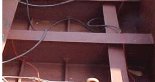
Fig. 6. Barge without Mastic
